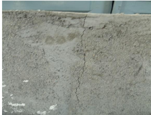
(c) Longitudinal crack in the bottom of the panel
