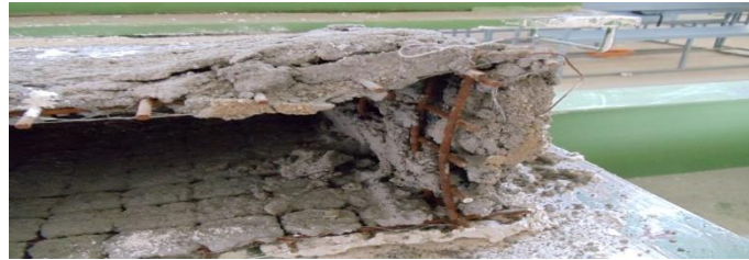
(b) Buckling of web reinforcement
