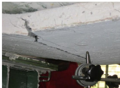
(b) Crack Across Thickness
