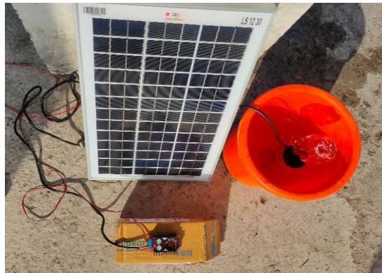
Figure 7. Solar PV based DC to DC Boost Converter for Water Pumping System
